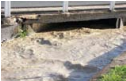
High energy water flows concentrated through culverts.
