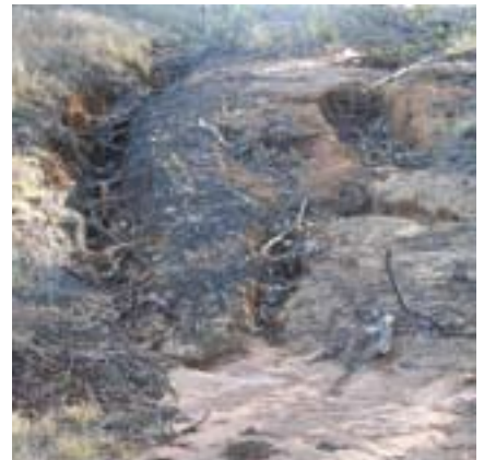
Gullies and Scour: Stock can produce tracks that can result in scouring and gully erosion on creek banks
