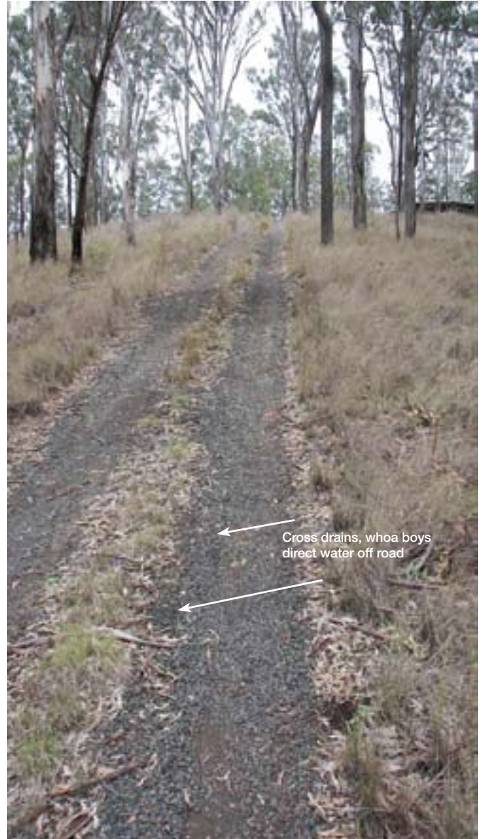
Basic erosion control – A steep track in the Helidon Hills area has been constructed on a ridge line with cross drains (whoa boys) to take water off the road to reduce erosion.
