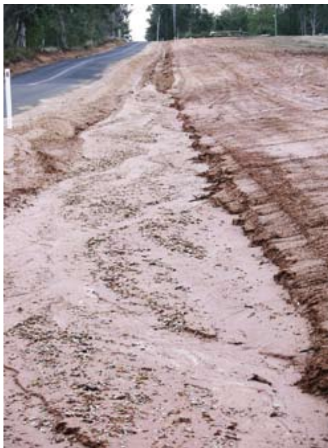
Sediment deposition from road erosion.
